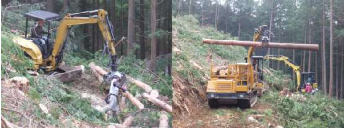
Photo 2 Chainsaw delimiting with grapple loader (Left) and Grapple loader loading to forwarder on a narrow strip road at Site B
